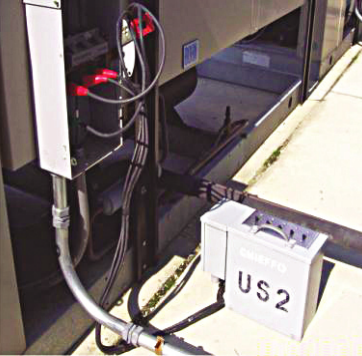
Optimizing refrigeration equipment
